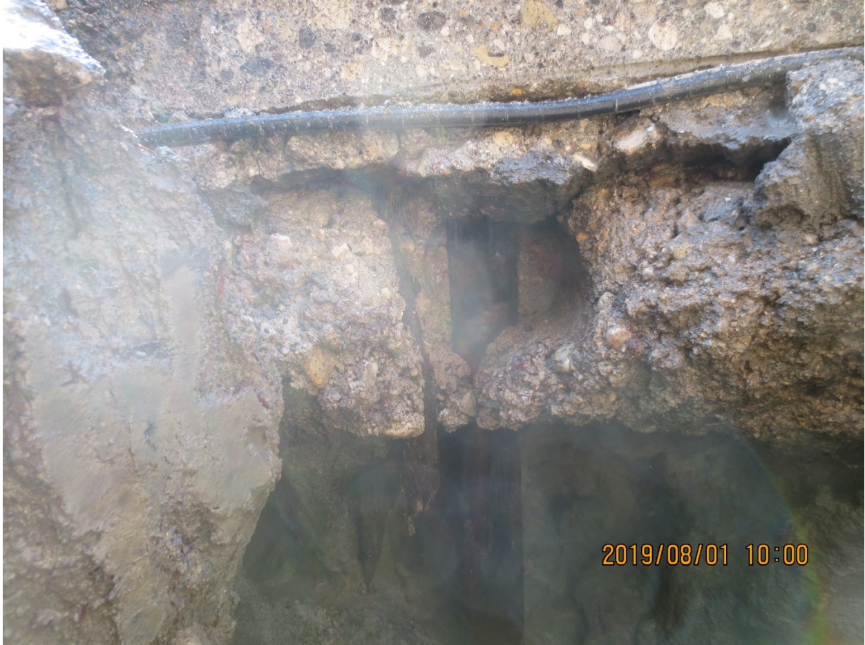
Figure 3 Streetcar Track Bedding below existing pavement (Station 2+360). Note previous wooden tie location.
