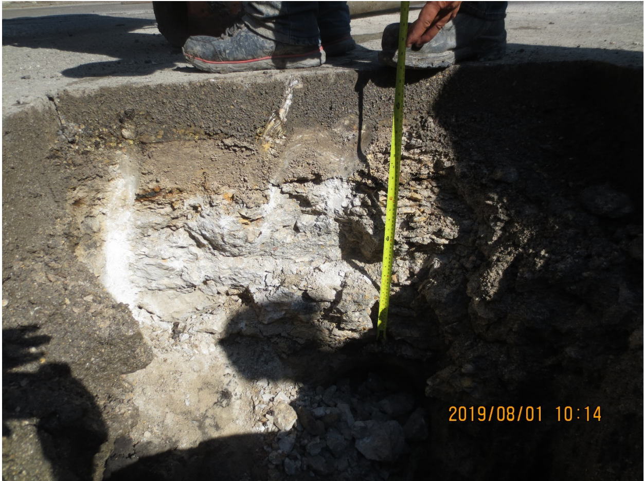
Figure 2 Streetcar Track Bedding below existing pavement (Station 2+360). The track bedding thickness measured 0.45m at this location.
